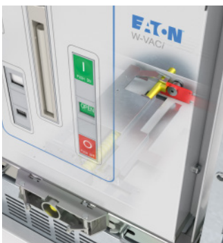
Racking mechanism interlock.
