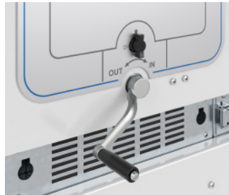
Racking behind closed door.
